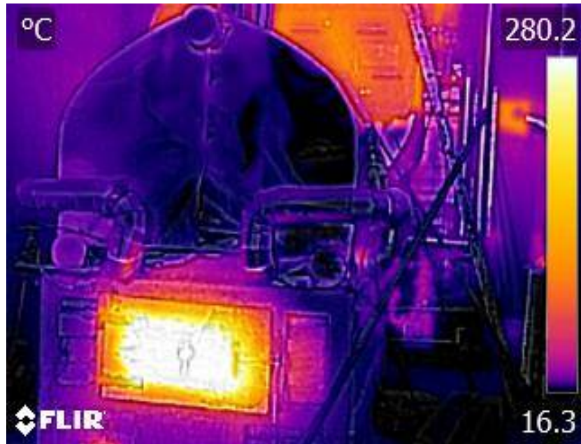
Heat losses following the poor isolation of the boiler door
